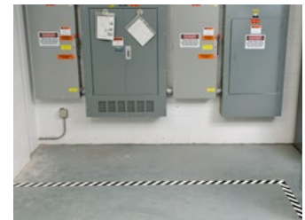
6. Colour-code areas in front of electrical panels.
