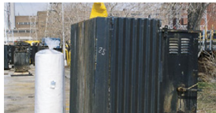
Ideal underneath leaking transformers.
