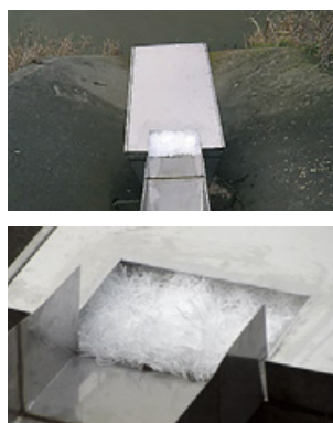
Filtering of waste water before discharging into water discharge area.
